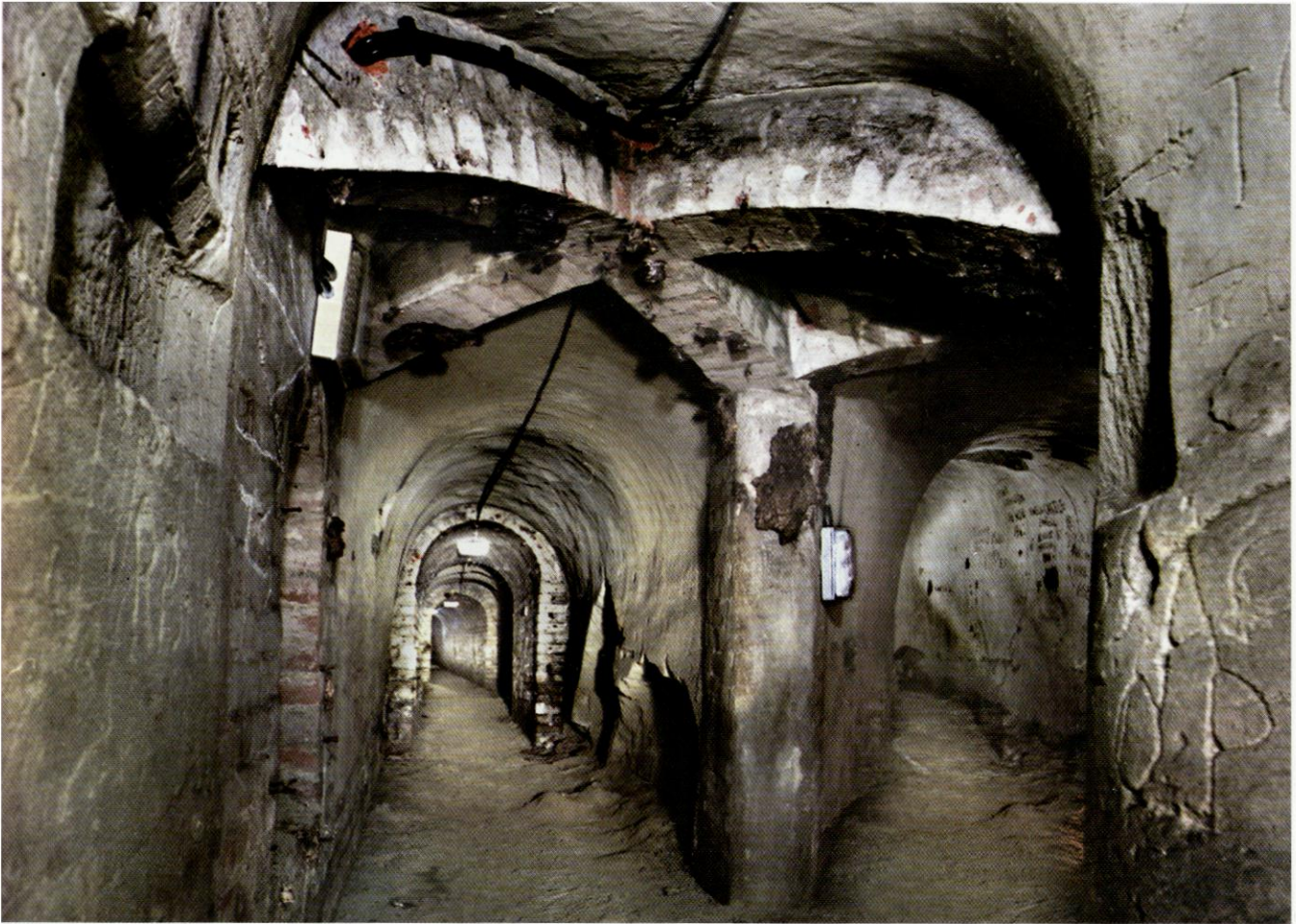
Looking north along the south tunnel beneath Ewell House in 1997. The branch to the right collapsed in 2001 and was subsequently backfilled. Note the vaulted buttressing found at many of the tunnel intersections. Photo: Nick Catford
